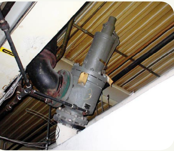
Safety valve is not installed vertically.
