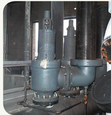
A proper safety valve installation with a drip pan elbow and proper drain lines off the safety valve and drip pan elbow.
