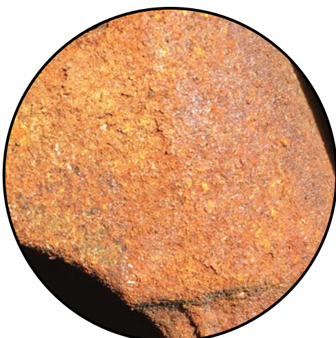
General (or Uniform) Corrosion
