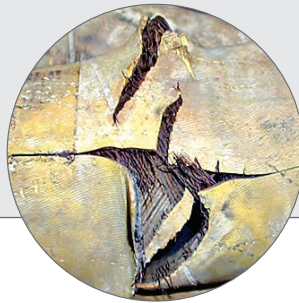
Excessive Cover Damage
