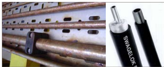
Figure 1. Corrosion of 316 stainless steel tubing in a typical offshore installation (left). Jacketed tubing and insulated jacketed tubing (right) may be wise choices in such environments.
