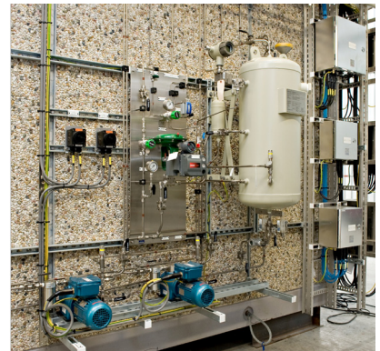
The gas vent recovery system built by Imtech Analyser Systems features Swagelok 60 series ball valves, R series proportional relief valves, regulators, variable area flowmeters, filters, and 40 series ball valves.
