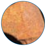
General (or Uniform) Corrosion
